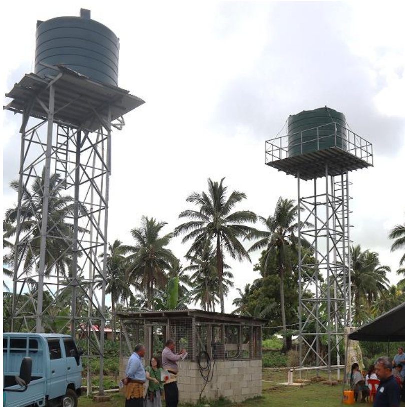
Water supply system for Tokomololo upgraded by Japan's GGP.
